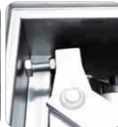
Mechanical gate stop inside the enclosure
