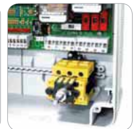
Detail of the disconnecter switch
